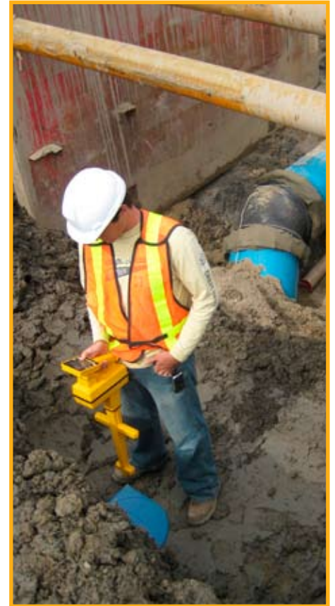
Many utilities, municipalities and water companies are beginning to use Radio Frequency Identification as a means to improve field operations.
